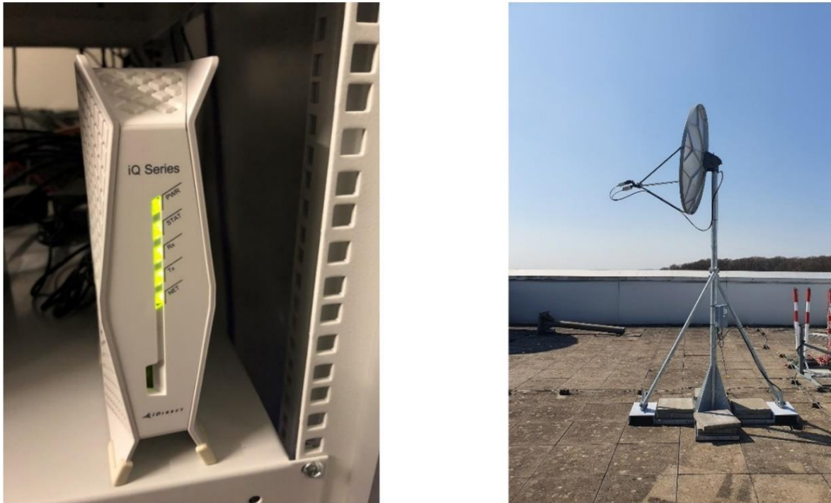
Figure 5: Fixed Edge Node installation at SES's Teleport in Betzdorf, Luxembourg: Out-Door Unit (ODU) + Indoor Unit (IDU)
