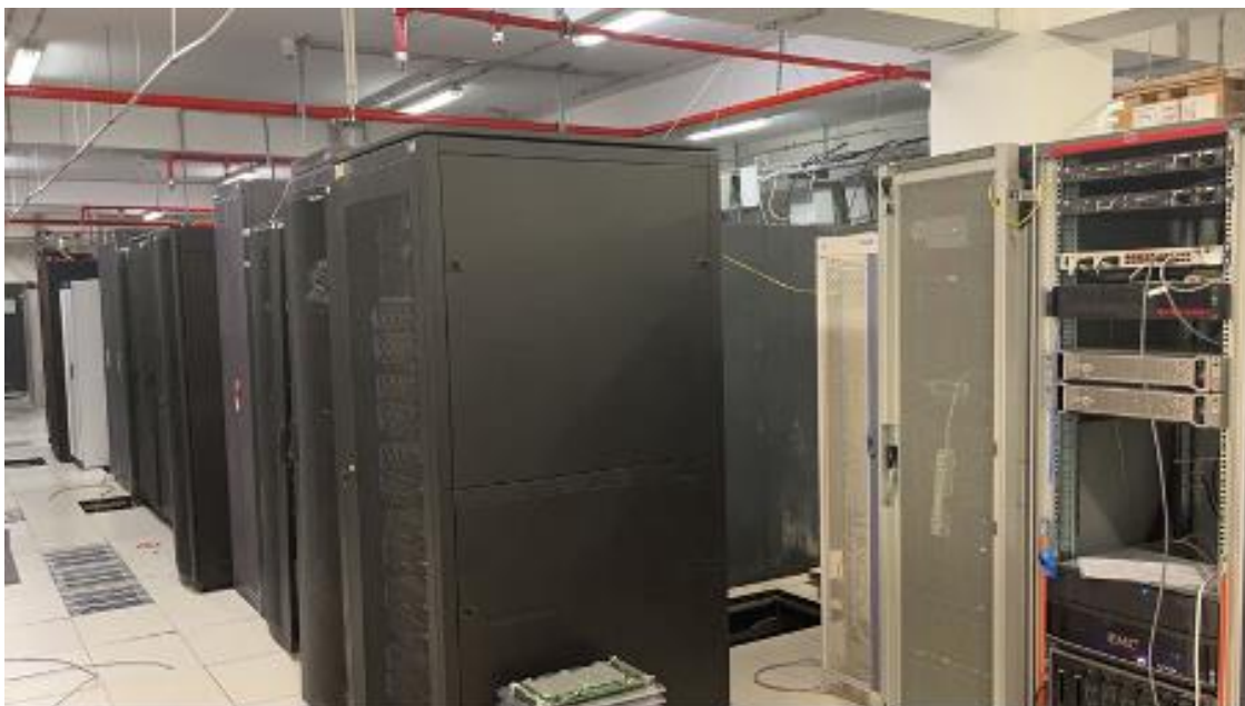
Figure 30: Turkcell IoT XG Test Platform System Room.
