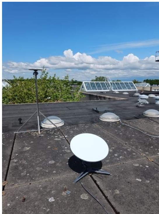
Figure 28: Starlink satellite UT in the roof of AAU 5G Smart Production Lab.
